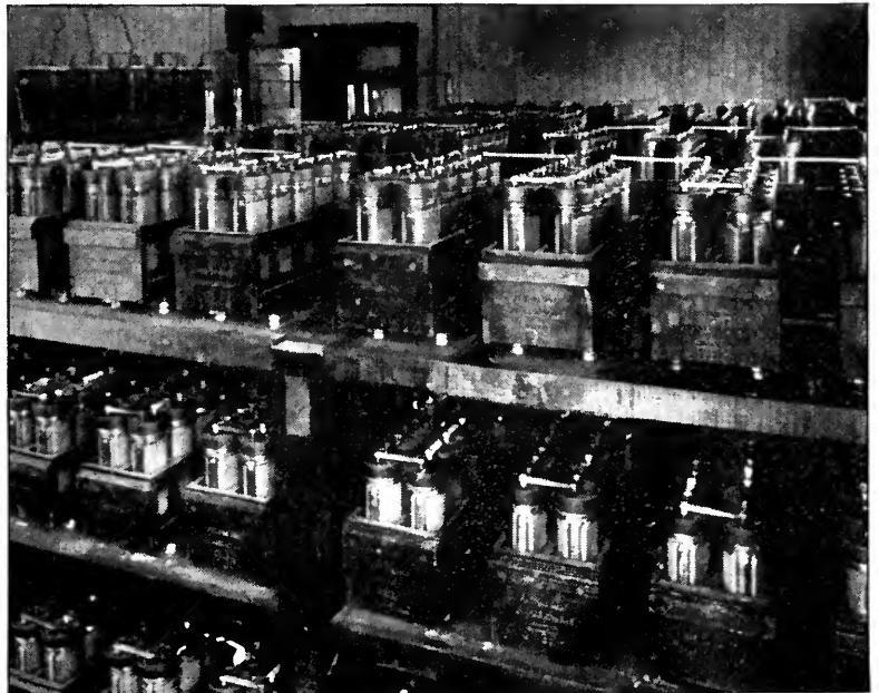
A FEW OF THE 1,400 BATTERIES THAT SUPPLY THE JUICE FOR WTAM Station of the Willard Storage Battery Company in Cleveland, Ohio
